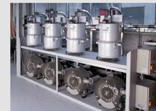
Central vacuum stations
